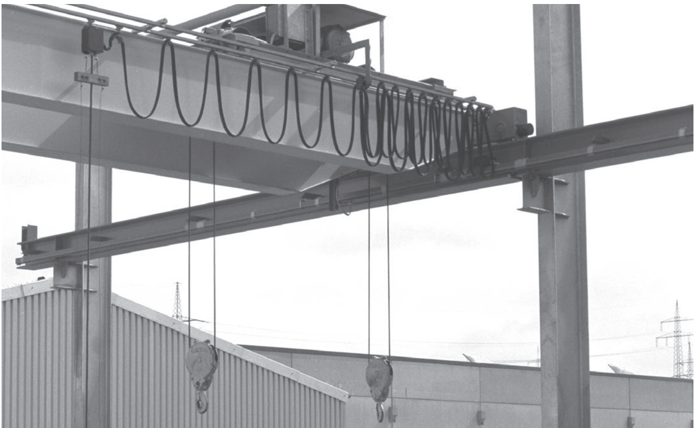
Cable carrier system for the cross travel on a outdoor crane
